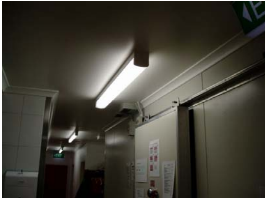
Picture 3: Light fitting with diffuser cover
