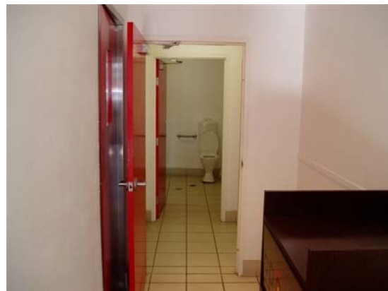
Picture 15: Toilets separated by air lock with self-closing doors
